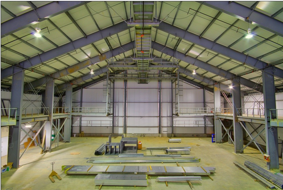
Illustration 6: Gateway Community Church, Abbotsford BC. Mid construction of a new State of the Art Modern Cathedral.
